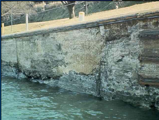
Crumbling lock wall, Lower Mon 3, opened in 1907
