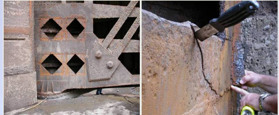
Miter Gate Cracking
