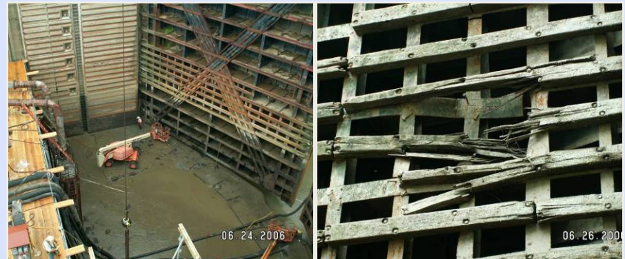
Dewatering & Gate Damage
