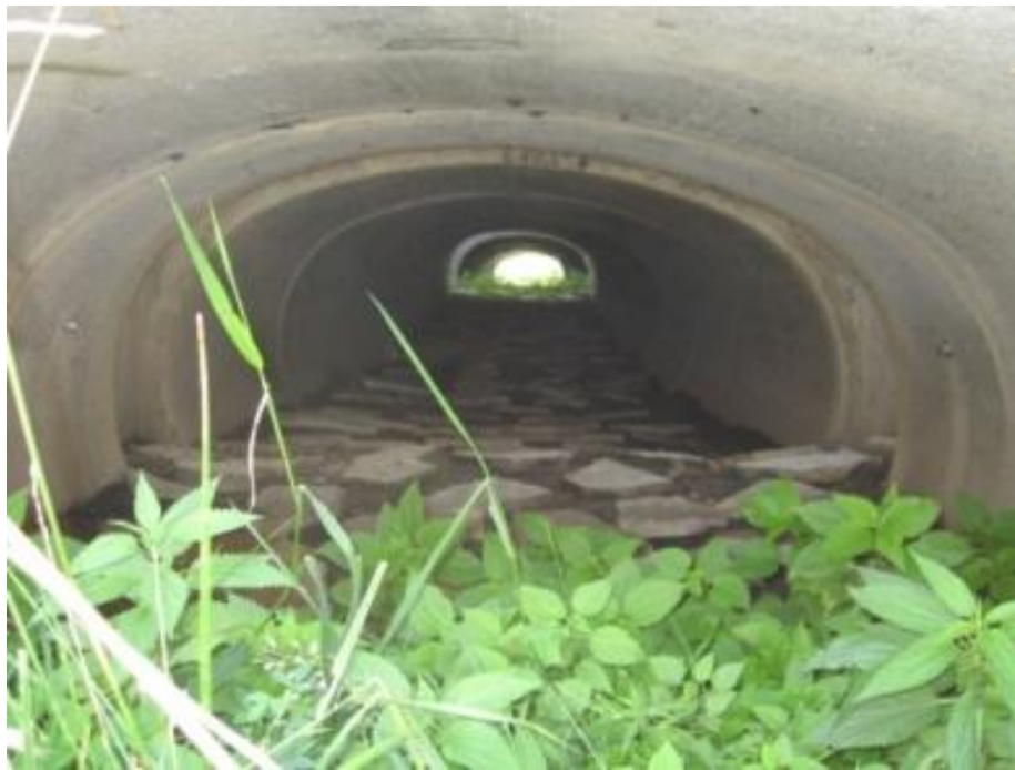
Figure 32 Ecopassage Condition, Summer, 2008 Photo Credit: Karla Leithoff, WisDOT
