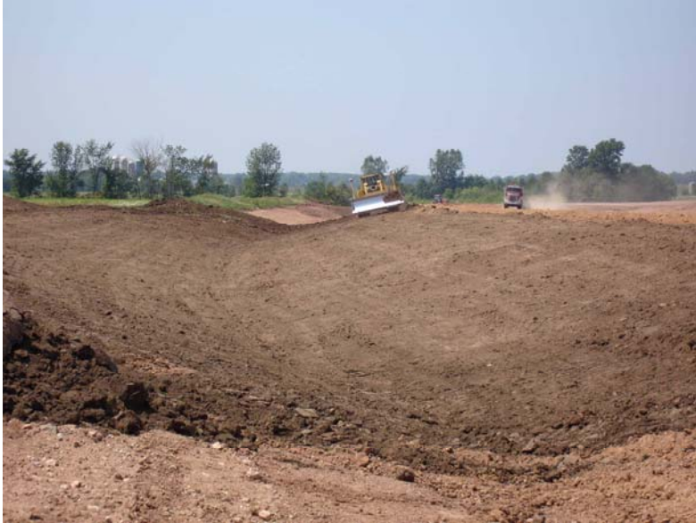
Figure 6. Slope and Ditch Work Using GPS Machine Guidance on the Mashuda Project
