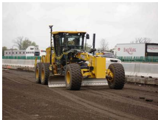
Figure 15. A Motor Grader Using TOPCON CORS-Based GPS Machine Guidance on I-94 Illinois Tollway Reconstruction (Corrections are being Received by Cellular Connection to a Central Server)
