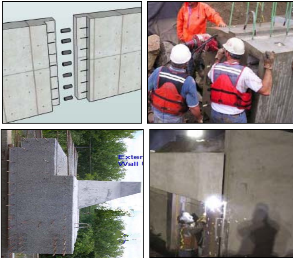
Figure 4 – Abutment module to module connection methods: Spliced Sleeves (top left), Post tensioning (6) (top right), Cast in place closure joints (7) (bottom left), Welding (8) (bottom right)
