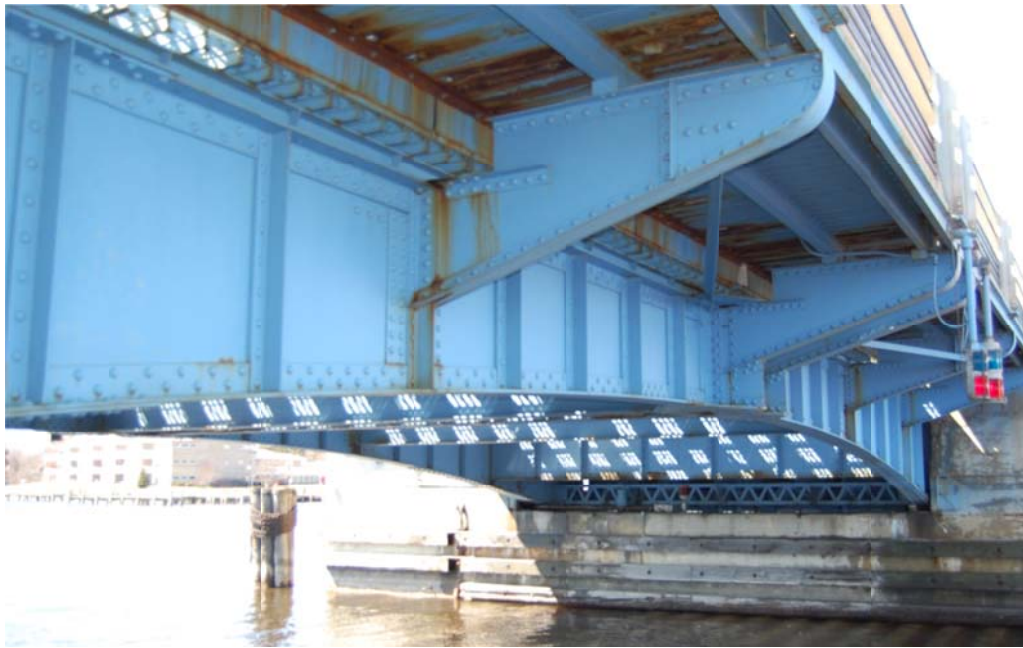
Figure 5.1-3. Bascule Girder view. Stiffeners every 3.6 ft. and a variable cross section along the bridge.
