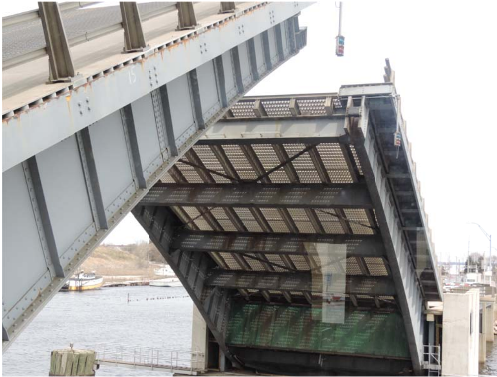
Figure 4.1-4. View of Marinette framing from below leaf and joint locking mechanism at the open end of the bascule girder.
