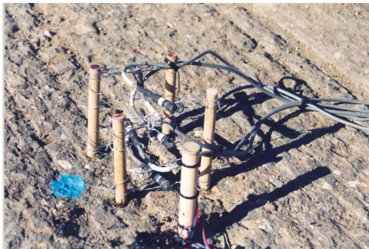
Figure 7.8: Relative humidity “Trees” installed at MnROAD
