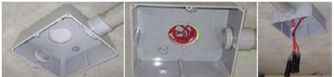
(c) Exposed Conduit, Wire, and Splicing.
