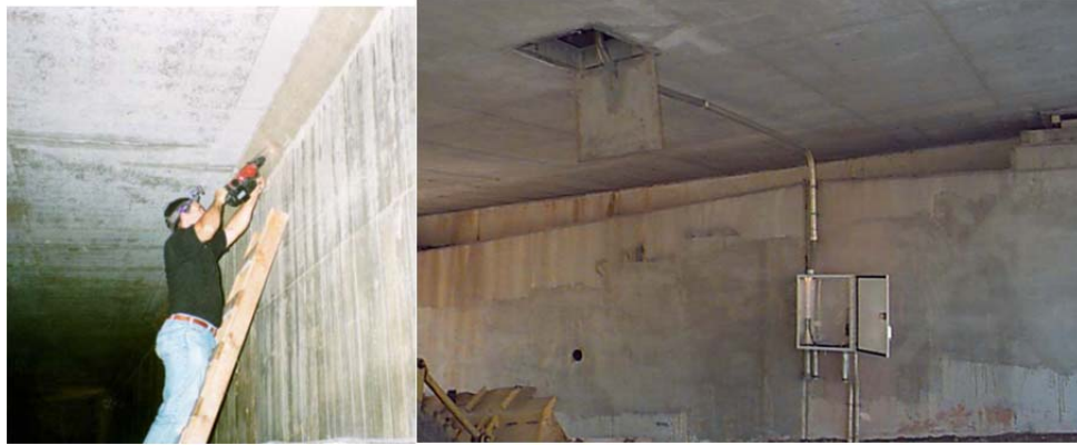
(a) Installation of temperature sensor (b) Enclosure for system control and cable conduit
