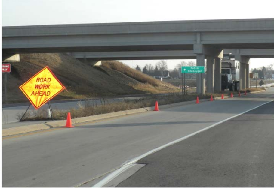
Figure 3.5. Site setup at DOT-10c with traffic control devices in the form of signage and cones.
