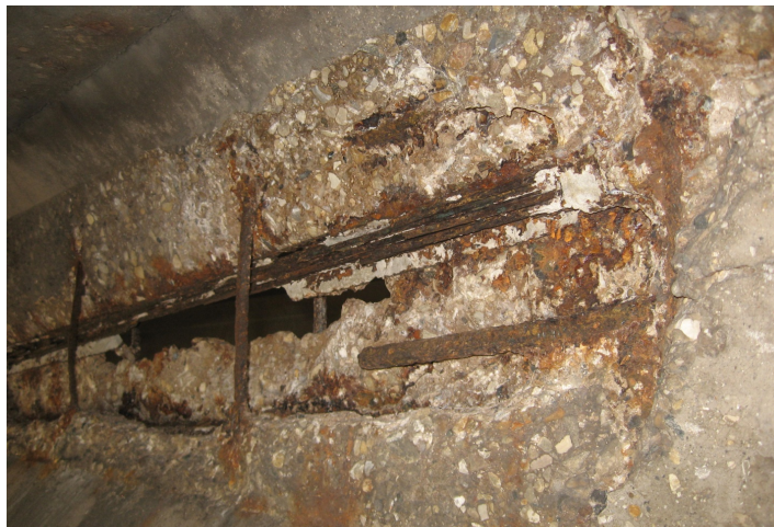
Figure-1. 1 Strand and rebar deterioration in US 45 bridge in Milwaukee
