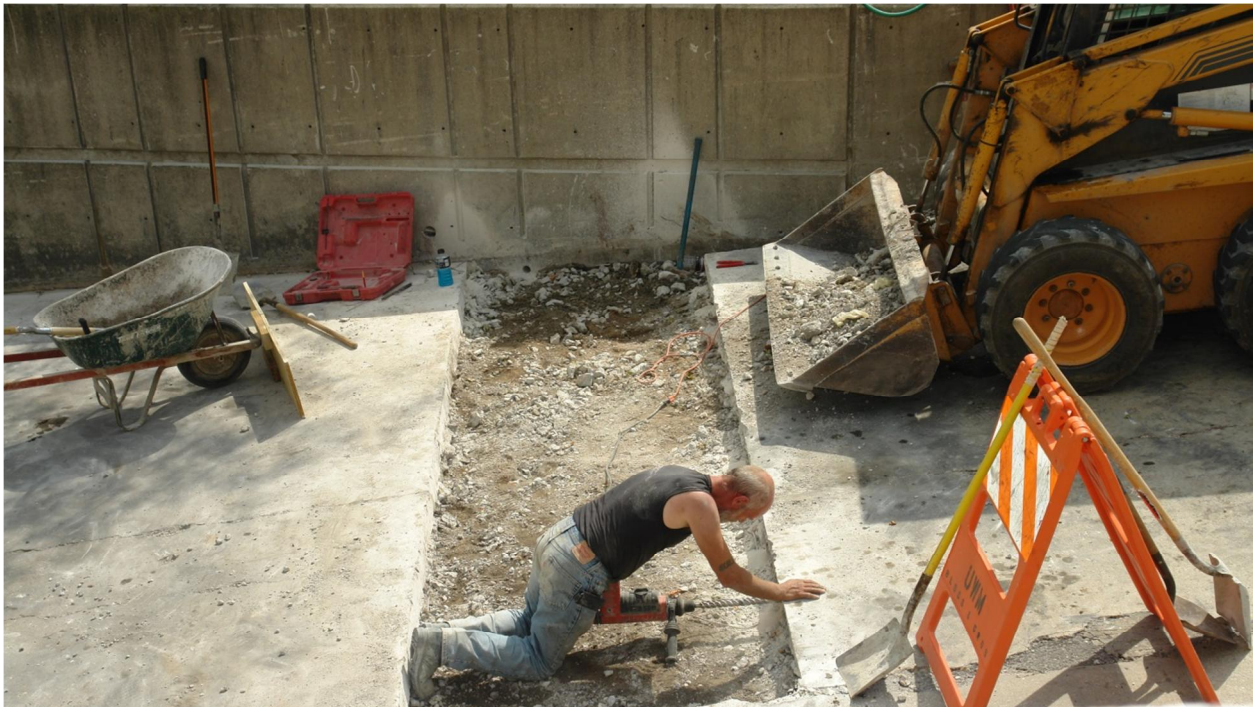
Figure 45: Drilling of the dowel bars for the SECC slab by the subcontractor
