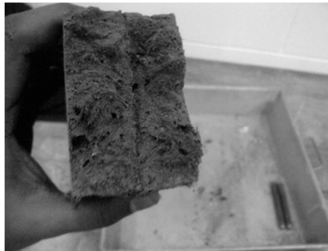
Figure 13: Cracks developed along the air voids in the interior of the beam
