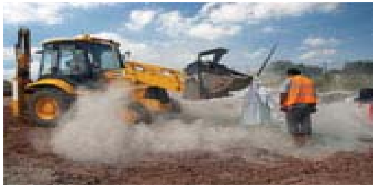
Recycled materials are increasingly used in base foundations for new or resurfaced roads
